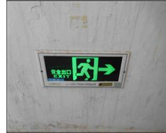
Photo of fire safety equipment Evacuation exit sign.JPG
