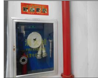
Photo of fire safety equipment Fire hydrant.JPG
