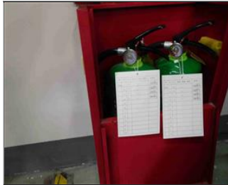
Photo of fire safety equipment Fire extinguisher.JPG
