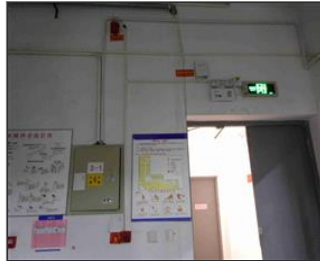
Photo of fire safety equipment Fire alarm Exit sign and Emergency light.JPG
